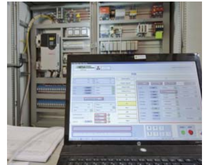
The electrical panel with a view on the PLC control system software.
